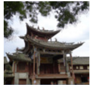
图9 云南沙溪寺登四方街古戏台 (修缮后) Pic. 9 Ancient performance stage on SidengSifang Street, Shaxi, Yunnan (After renovation)
